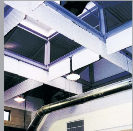
SONEX® One baffles in music room
