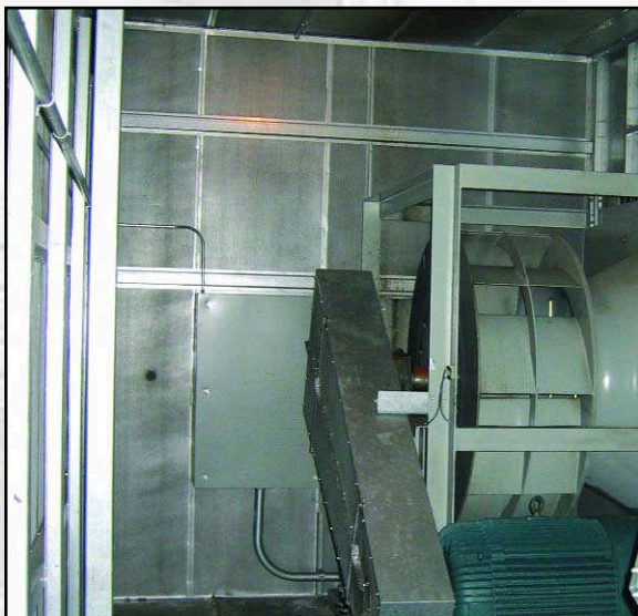
AHU Plenum Interior
